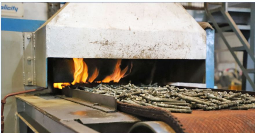
Heat Treatment Plant
